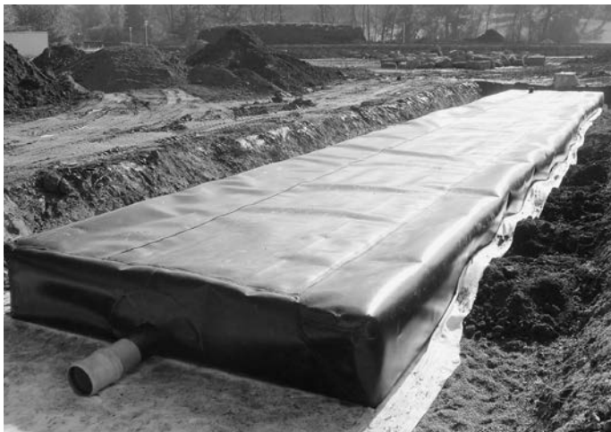
Rainwater tank with foil cover
