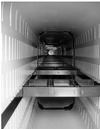
RAUSIKKO Box cleaning and distribution channel
